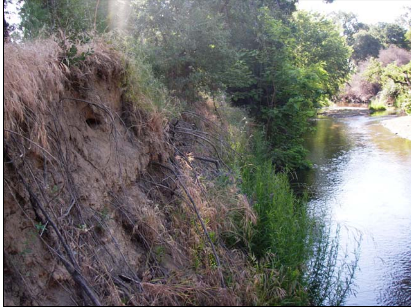
Description: Bank erosion at Dry Creek WWTP, E aspect
