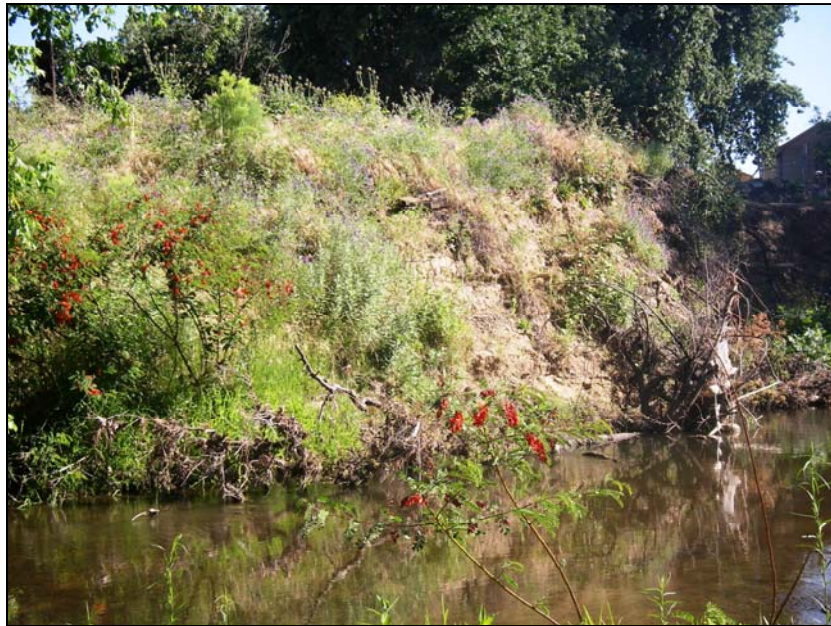
Description: Bank erosion at Dry Creek WWTP, N aspect (note Red Sesbania growing on both banks).
