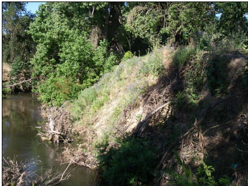
Description: Bank erosion at Dry Creek WWTP, W aspect
