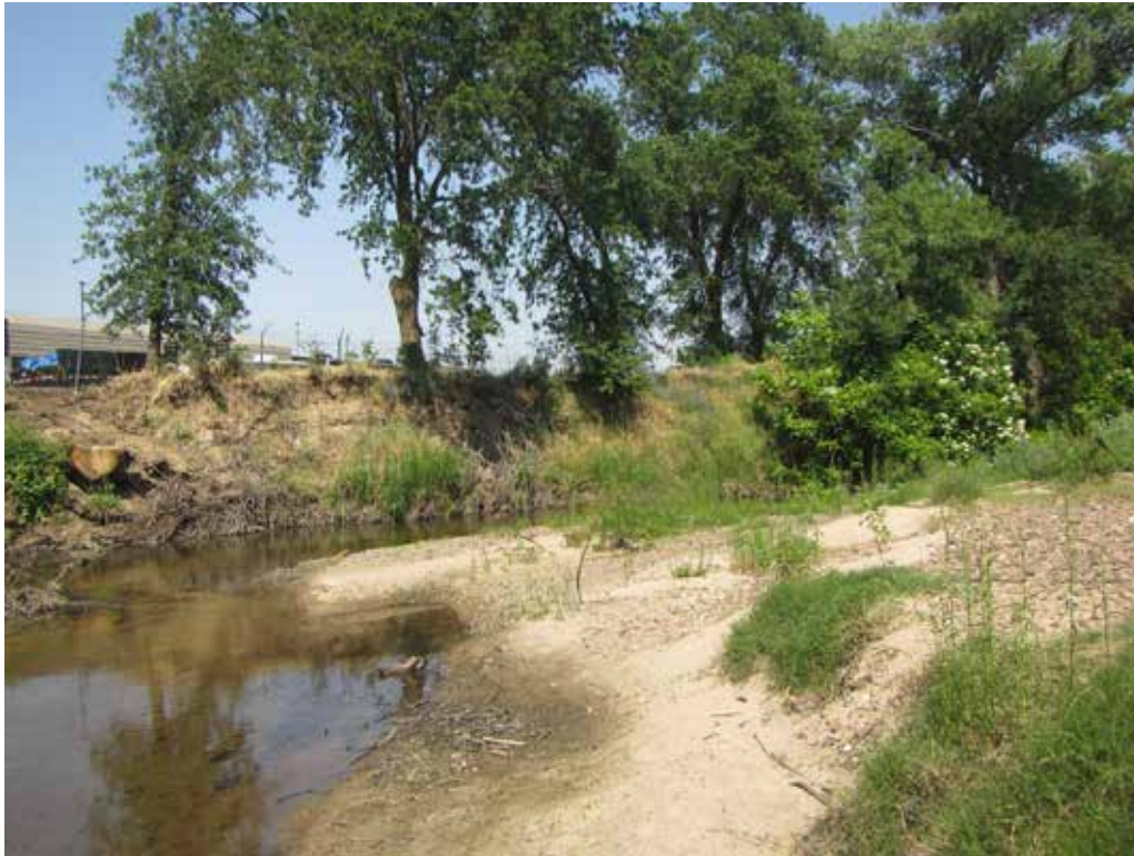
Photo 1. Near vertical bank with trees located 1,070 feet upstream of the Dry Creek WWTP (at the Booth Road Site). The Oak Trees are about seven to eight feet from the sewer and if the trees fall, they will put the sewer at risk.
